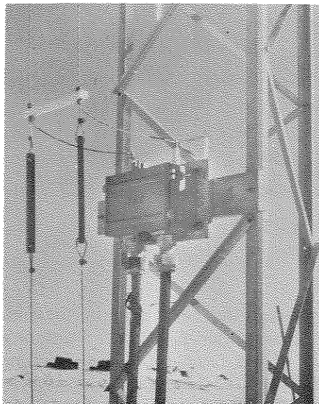
BAC-2 BEVERAGE ANTENNA COUPLER
