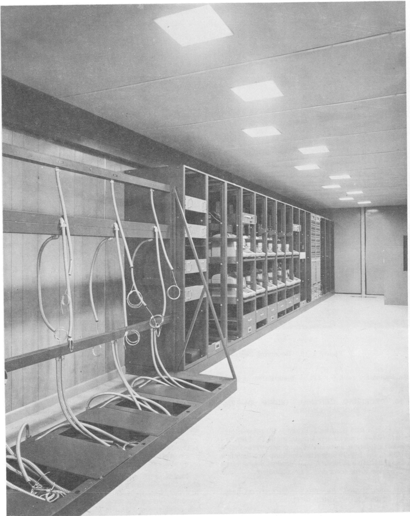
Figure 1-11. Teletype Central AN/TGC-16 (RB1, Equipment Installation)
