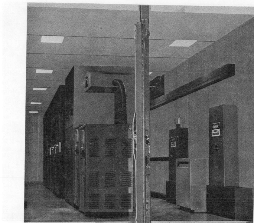
Figure 1-52. Radio Transmitting Set AN/TRT-25 (TH4, 50-K Installation, Front Area)
