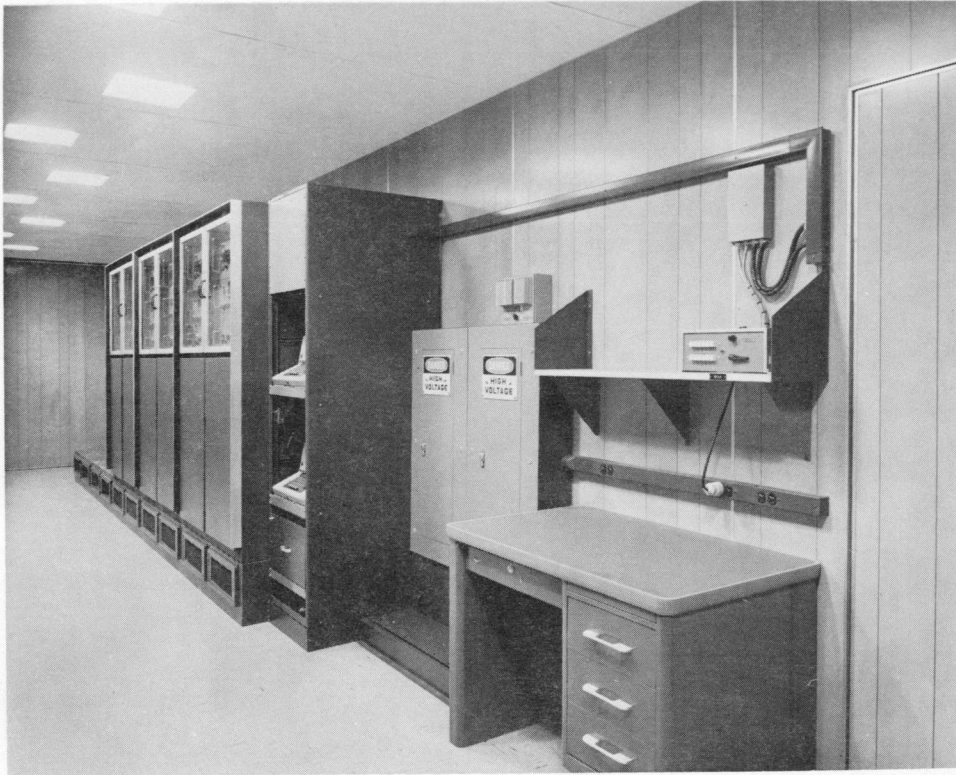
Figure 1-23. Receiving Central Group OA-4944/TSR-1, (RE3, Right Side Equipment)
