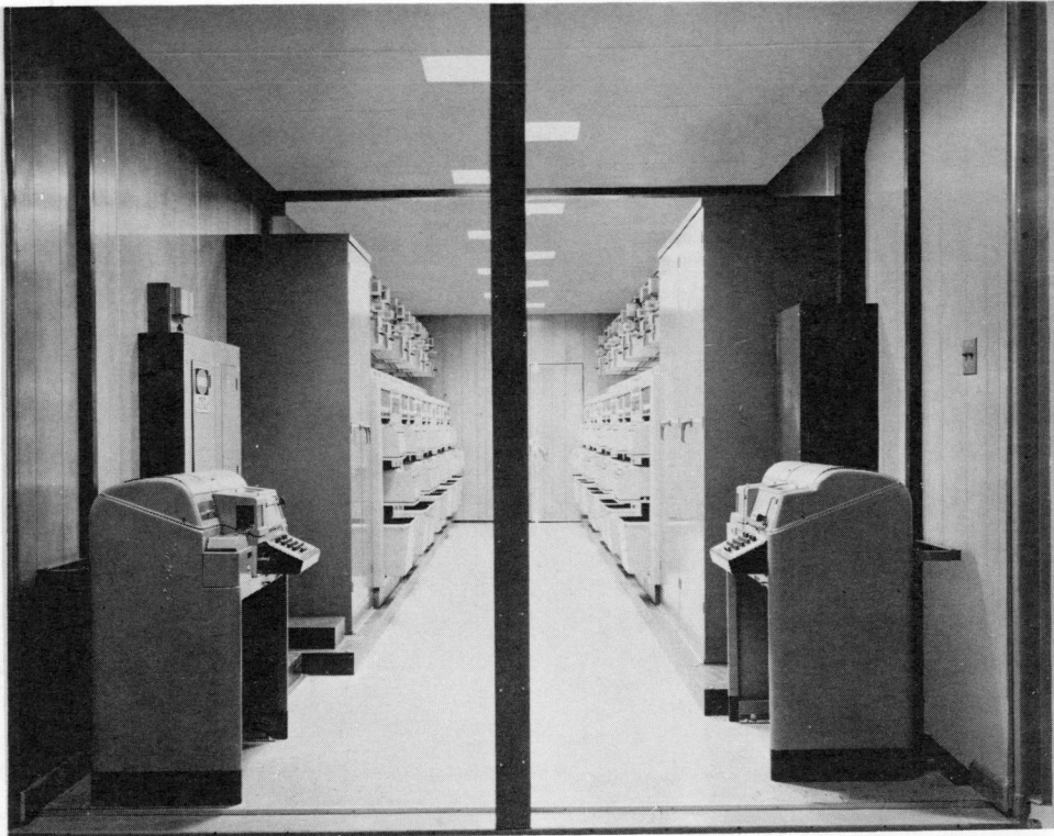
Figure 1-36. Teletype Central AN/TGC-19 (RJ2, Equipment Installation)
