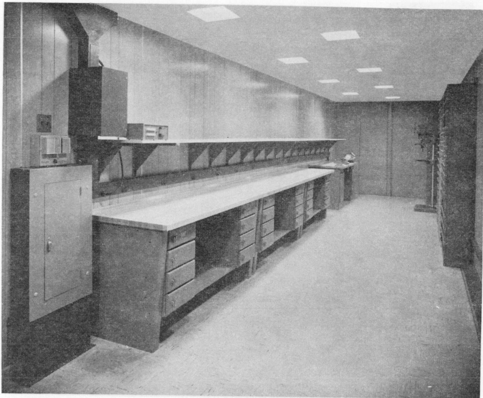
Figure 1-17. Maintenance Equipment Group OA-4941/TSR-1 (RD1, Equipment Installation)
