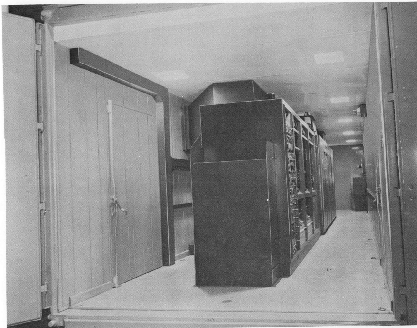
Figure 1-49. Radio Transmitting Set AN/TRT-24 (TH3, 200-K Installation)
