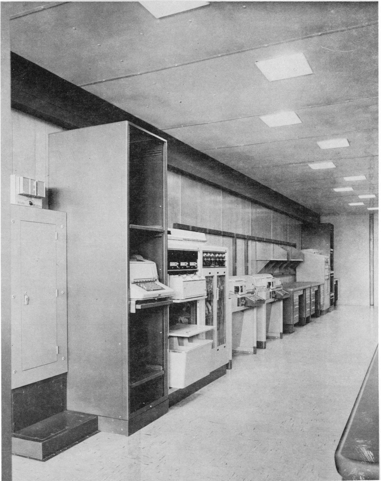
Figure 1-26. Receiving Central Group OA-4945/TSR-1 (RF1, Left Side Equipment)
